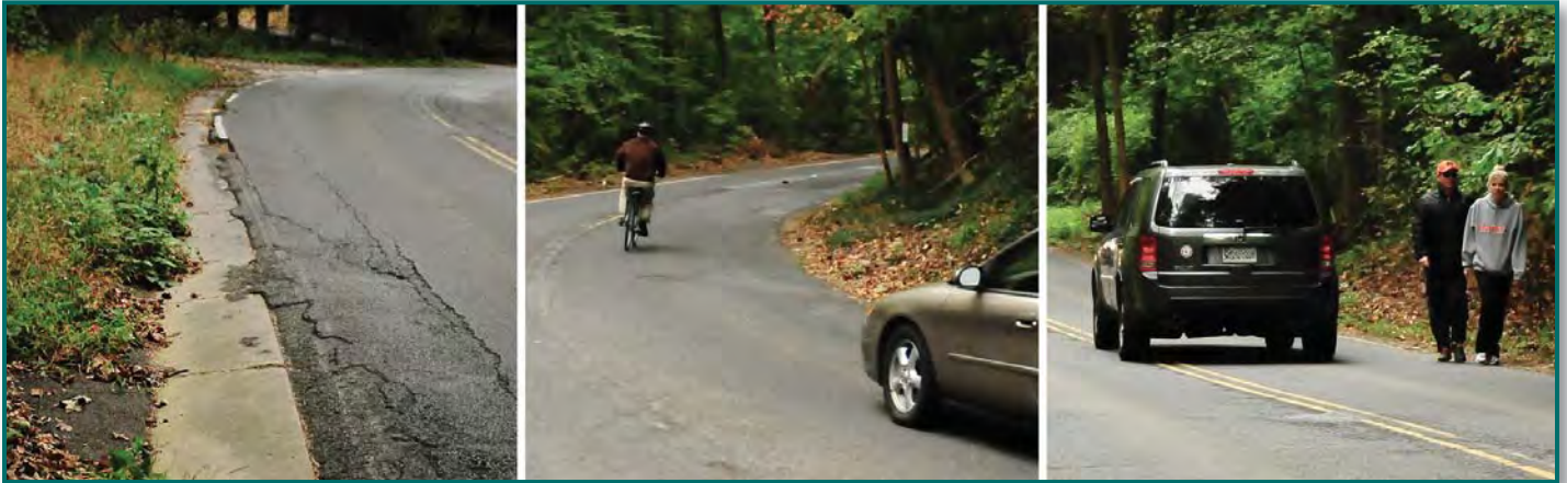
The existing roadway has deteriorated pavement and poor drainage and lacks safe means for bicyclists and pedestrians.
